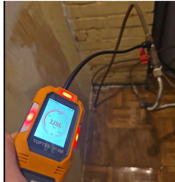
Gas leak found
